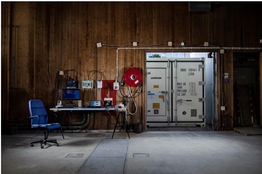
Fig. 2 – CNC-control desk and the refrigerated 20' container
